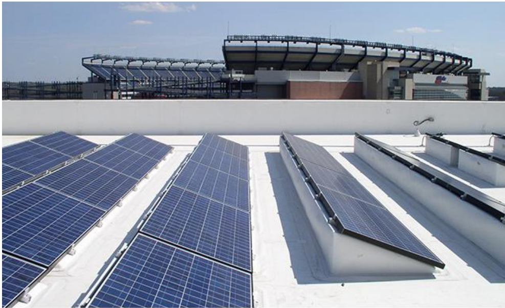
Patriot Place Solar Installation (Photo by Chris Bills)
