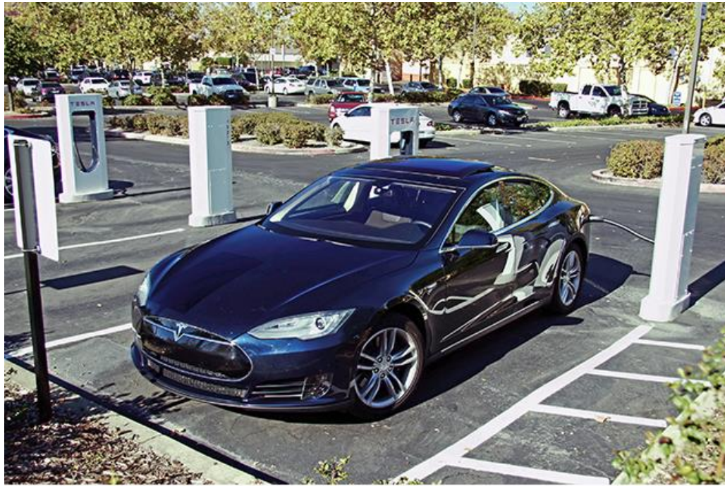
Electric Car Charging Station in California (Photo by Mariordo)
